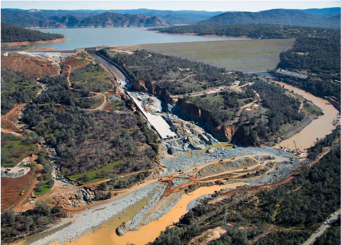
Figure 13-5. Oroville Dam Emergency Spillway Failure in Spring 2017
