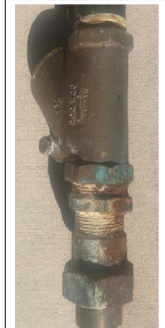
Corrosion on riser
